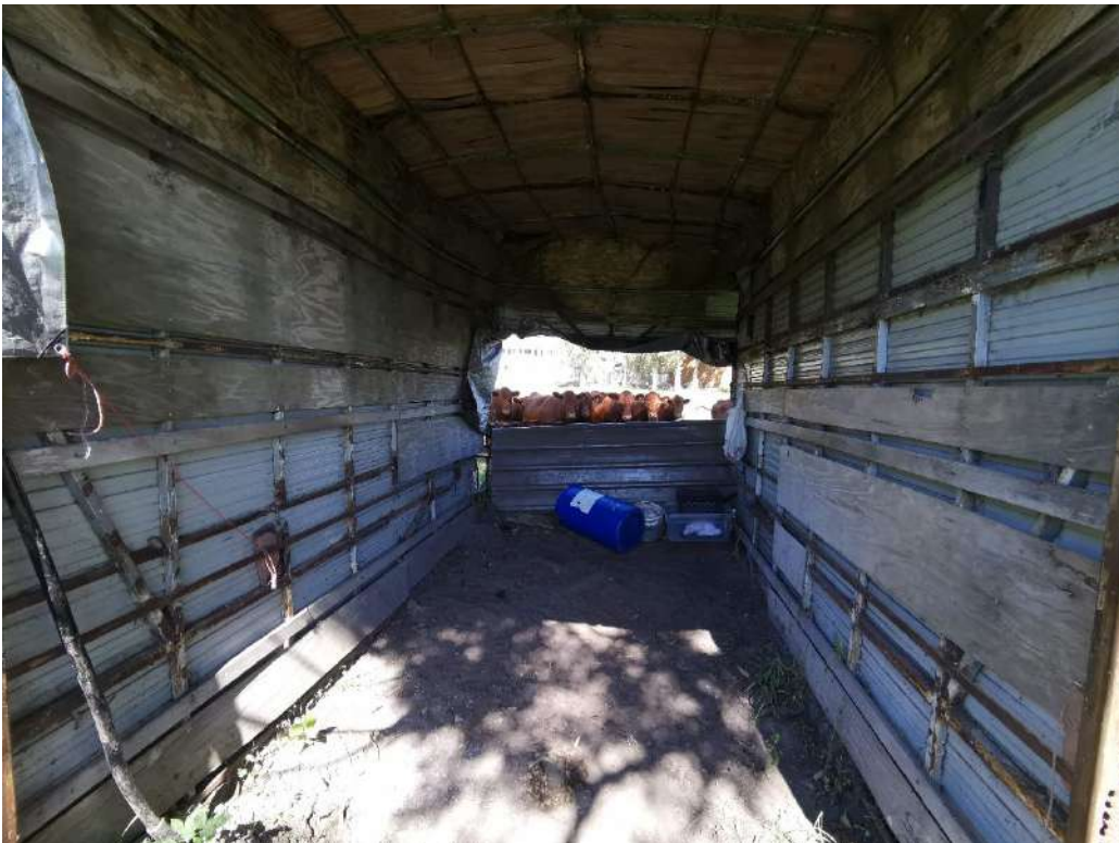
Photo 4.14 Inside of a portable shed/animal shelter, west of the site access driveway (now completely dilapidated)
