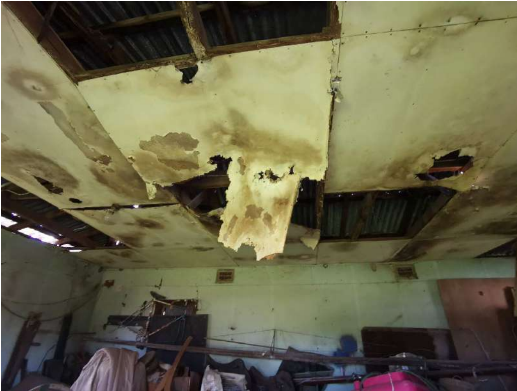
Photo 4.13 Existing storage shed attached to the stables showing state of structural decay
